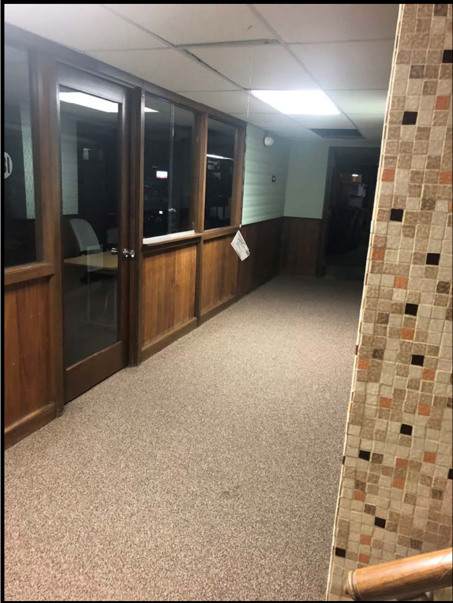
Photo B10 - Looking east near the west stairs exit of the basement. Remove and dispose of all carpeting in basement. This includes the adjacent Teller / Bank Vault Room.
