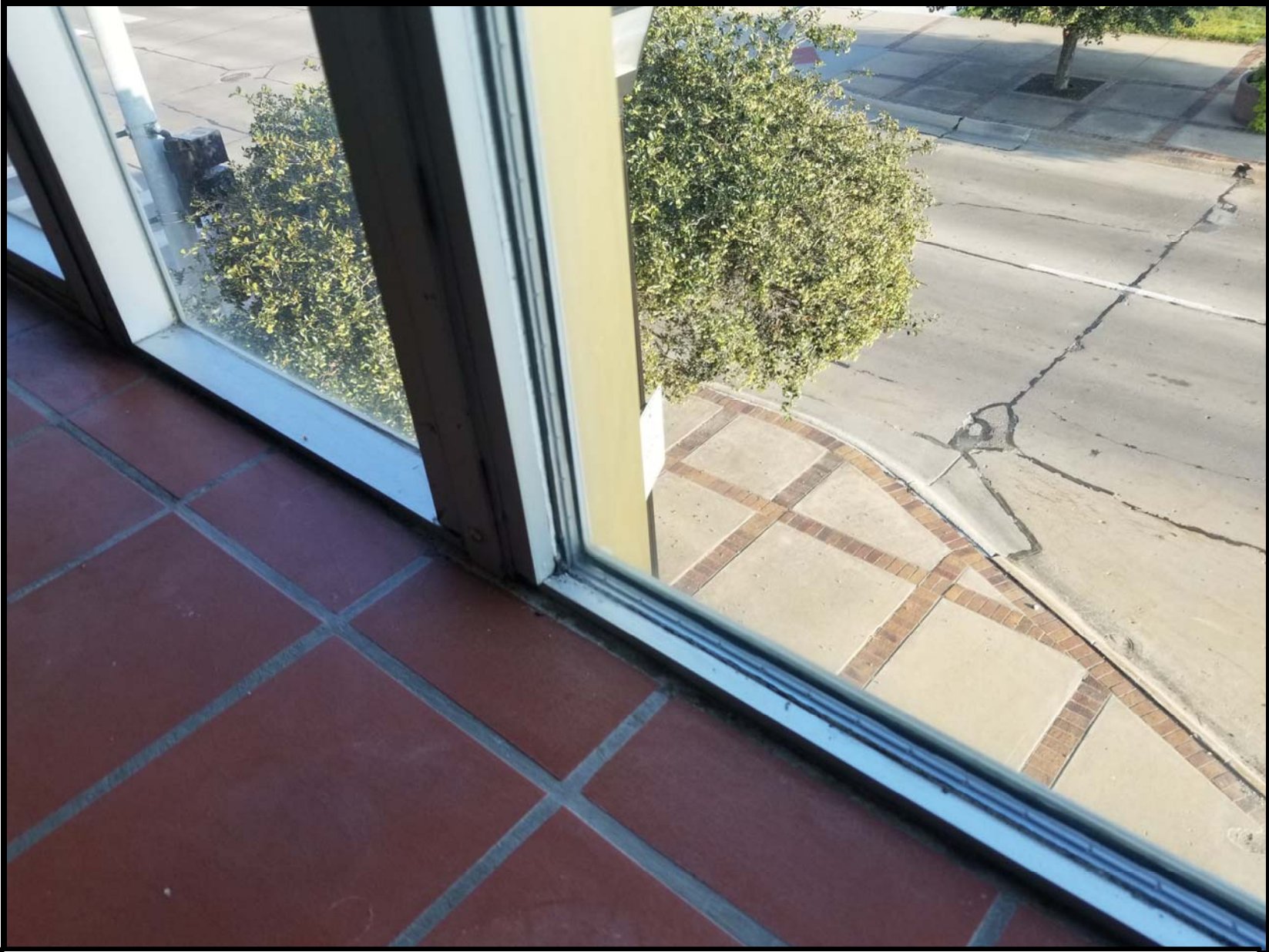
Photo SF8 - Looking northwesterly towards the bottom of a window on second floor. Remove all ACM caulking as required and as noted in Quad-C ACM report. Remove and salvage all curtains to properly remove ACM.
