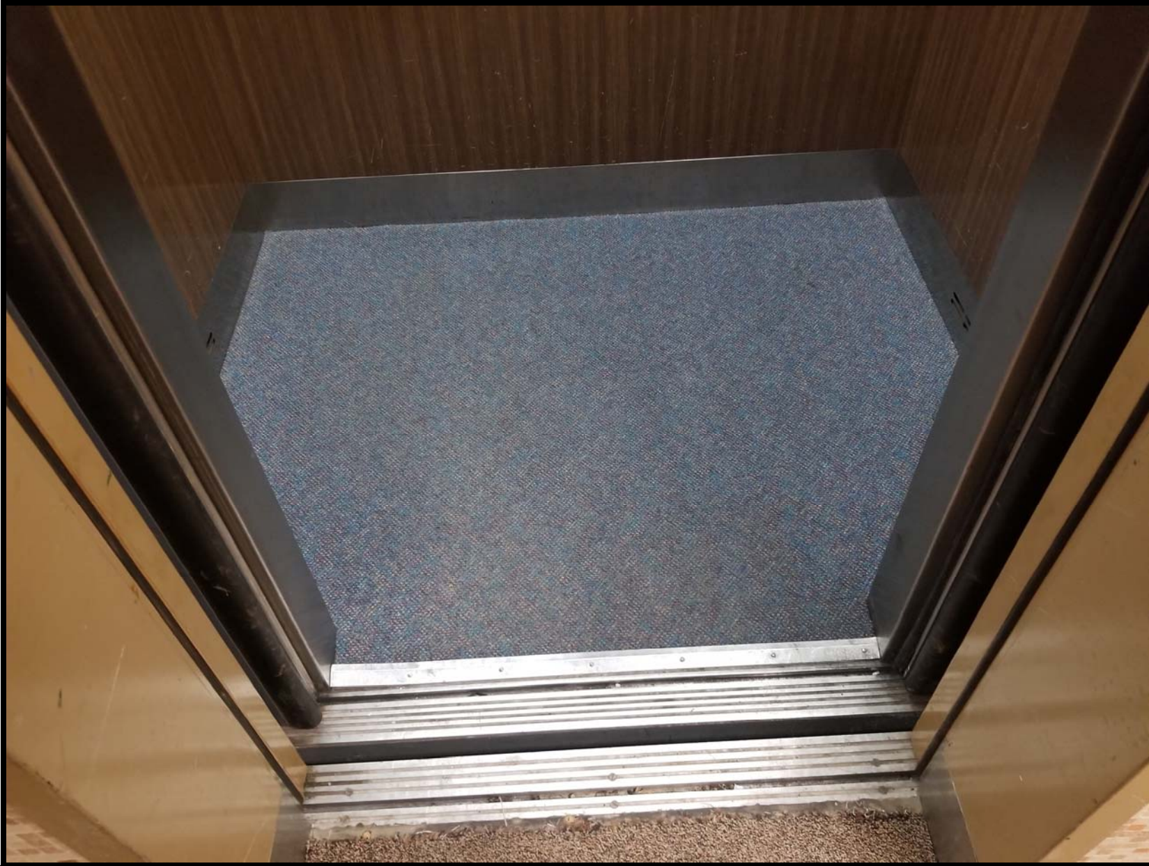
Photo B8 - Looking south into the elevator car. Remove and dispose of carpet.
