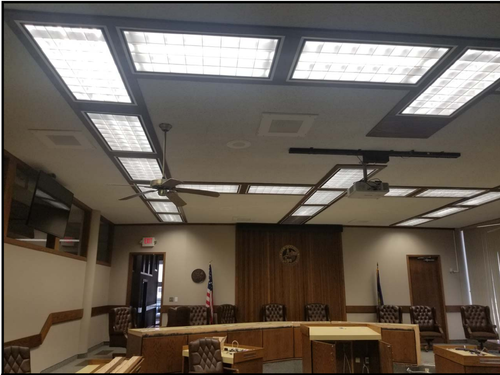
Photo FF5- Looking west from the east end of the council chambers located on first floor. Remove and abate ACM ceiling texture. Remove and dispose of all crown molding ACM, light fixtures, speaker assemblies, air vents and ceiling fans required to properly remove ACM.
