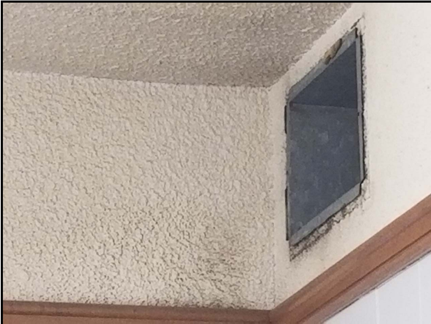
Photo SF5 - Looking northerly within the office located on the northeast end of second floor. And Remove and abate all ACM ceiling and wall texture. Remove and dispose of all light fixtures required to properly remove ACM. Remove and salvage all wall molding required to remove ACM. Remove and abate all mold found on ceiling and wall substrate.
