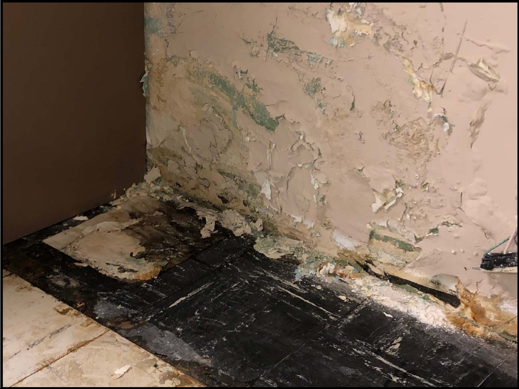
Photo B5 - Looking north towards the outside basement wall northwest of the basement kitchen area. Remove and abate all mold. Remove surface of soft concrete areas that cannot be properly abated for mold.
