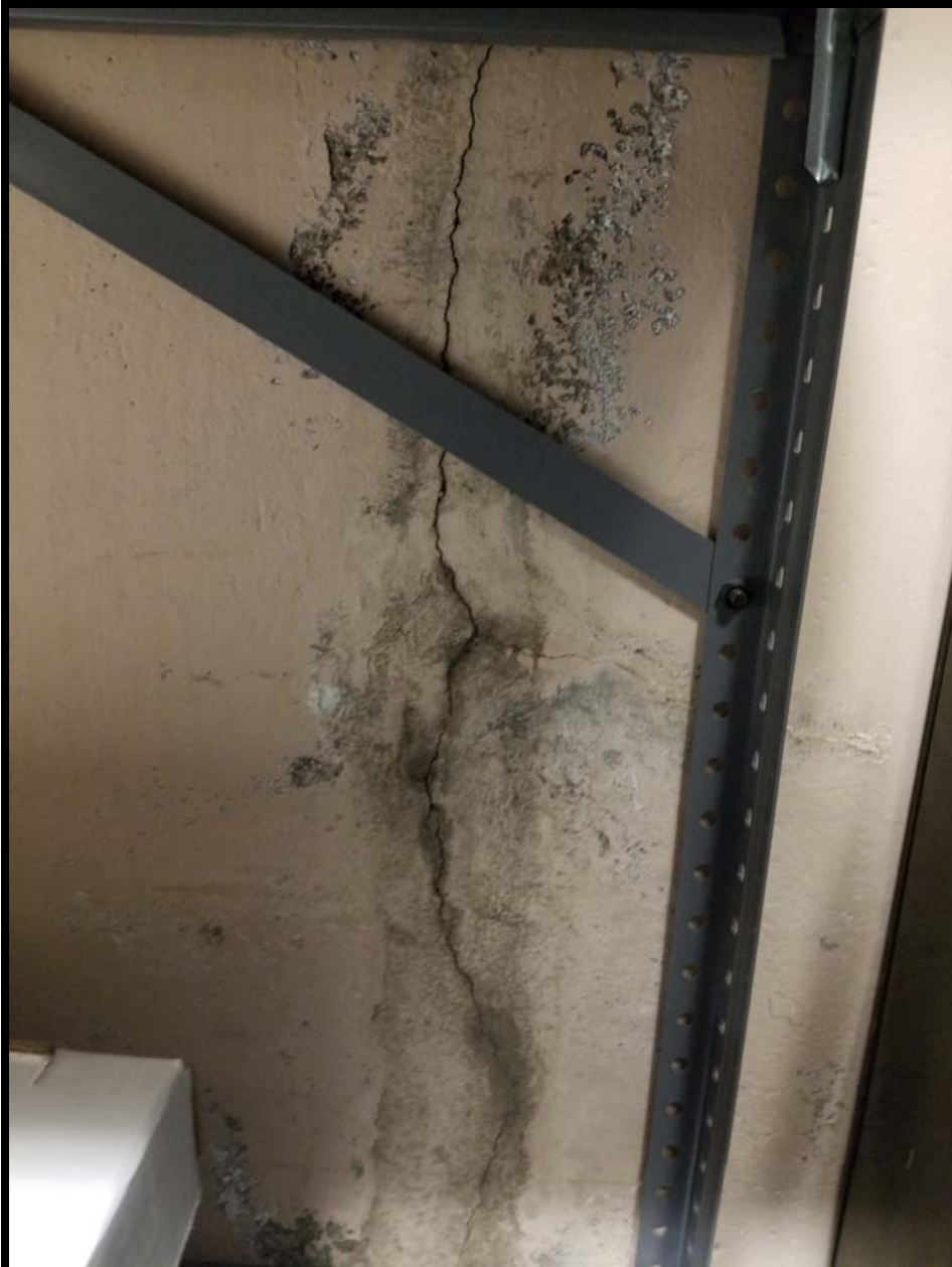
Photo B2 - Looking south from near the southwest corner of the basement. Remove mold and abate surface.
