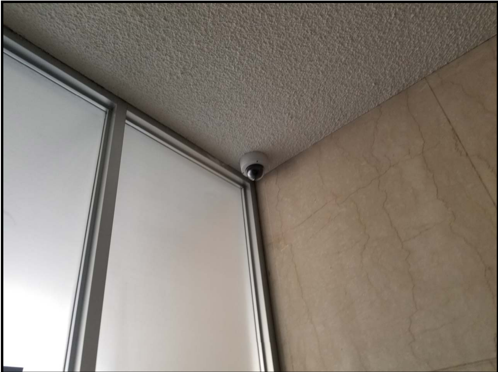
Photo FF1 – Looking northwest towards security camera located in the west first floor foyer. Additional camera in southeast corner of the foyer. Remove and abate ACM ceiling texture. Remove and salvage security camera to properly remove ACM. Typical all security camera locations required to be removed to abate ACM shall be salvaged.
