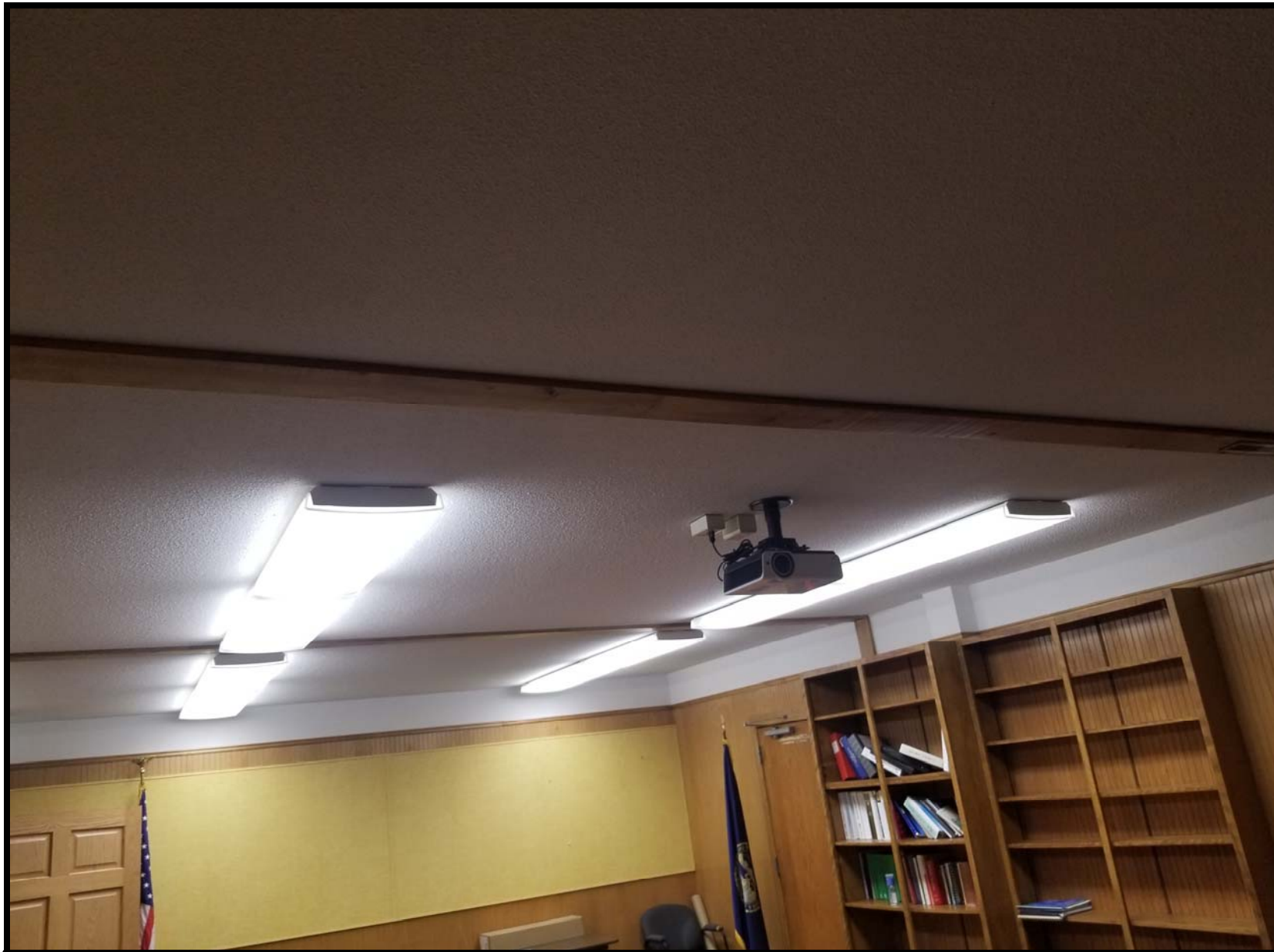
Photo SF4 - Looking west within the main conference room of second floor. Remove and abate all ACM ceiling texture. Remove and dispose of all light fixtures required to properly remove ACM. Remove and salvage projector and screen. Remove and salvage wood molding required to properly remove ACM. Remove and dispose or reset electric service boxes to properly remove ACM.
