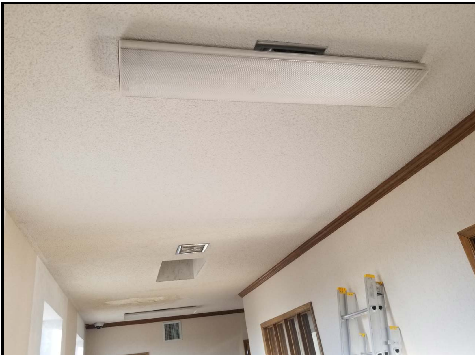
Photo SF1 - Looking south within the east end of the second floor hallway
