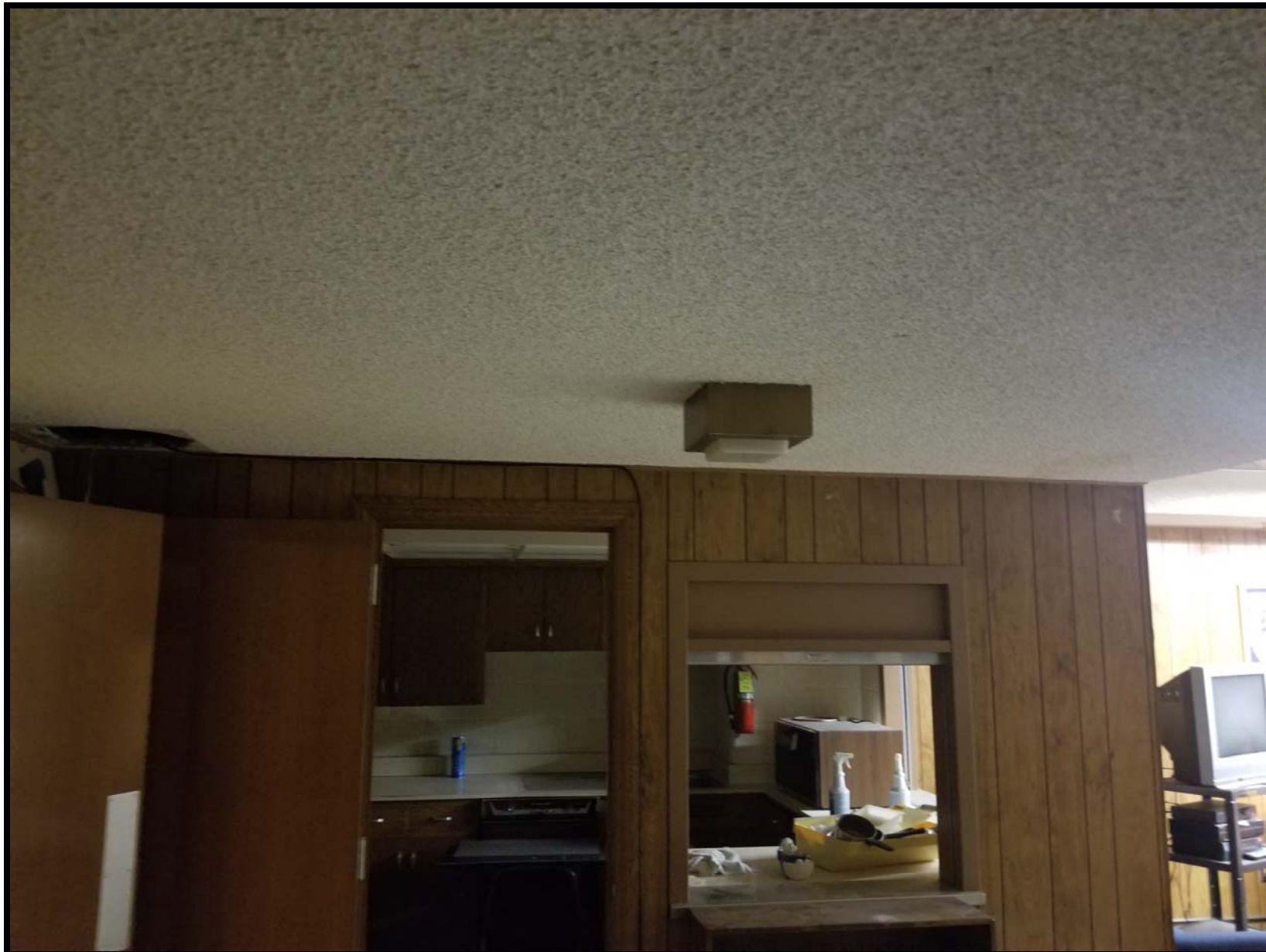
Photo B4 - Looking south near the north side of the kitchen area located in the basement. Remove ACM ceiling texture. Remove and dispose of all light fixtures required to properly remove ACM. Remove and dispose wall paneling and trim as required to abate ACM abutting wall paneling
