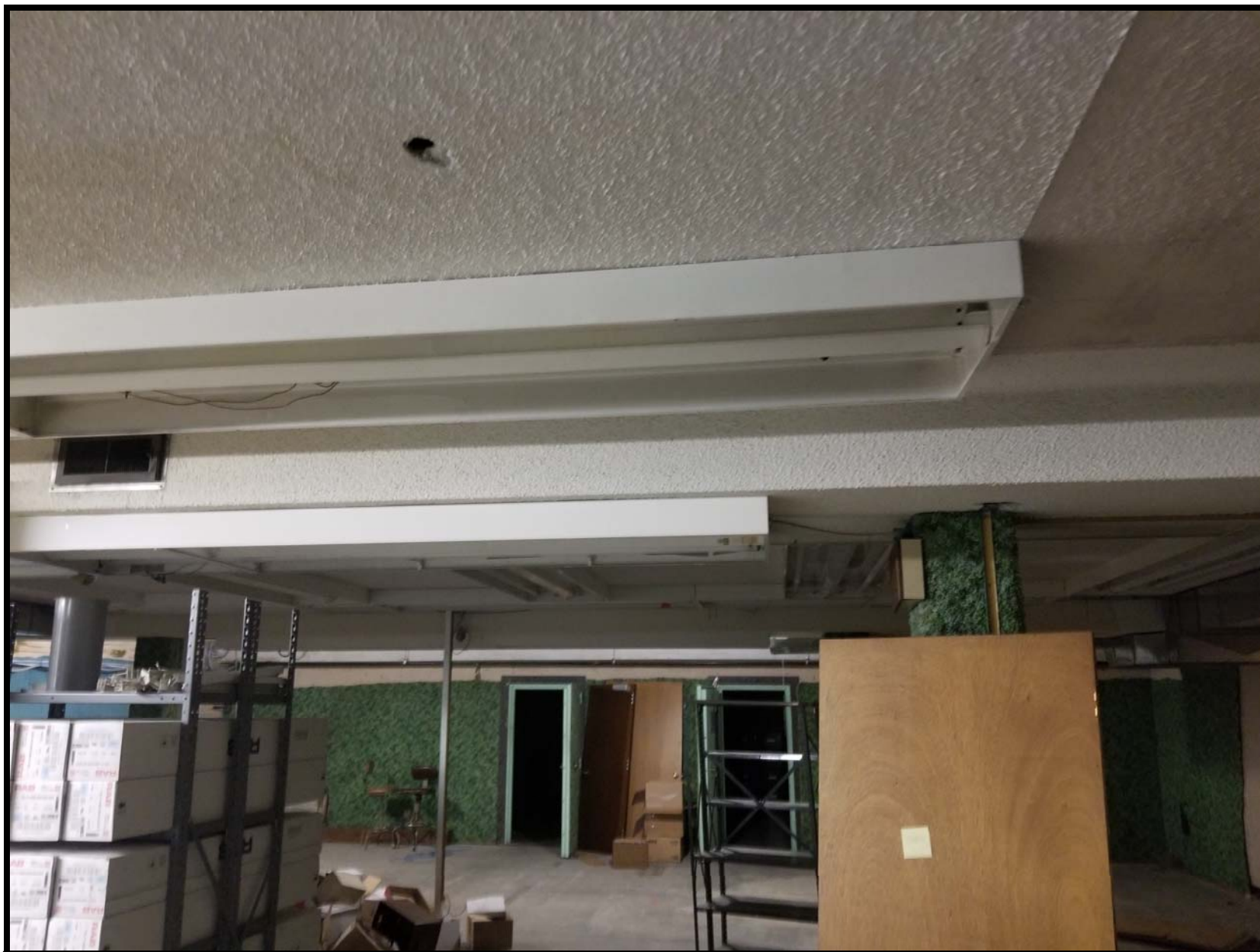
Photo B12 - Looking south within the main room of the basement. Remove and dispose light fixtures and vents required to properly remove ACM. Typical of all ceilings requiring ACM abatement.
