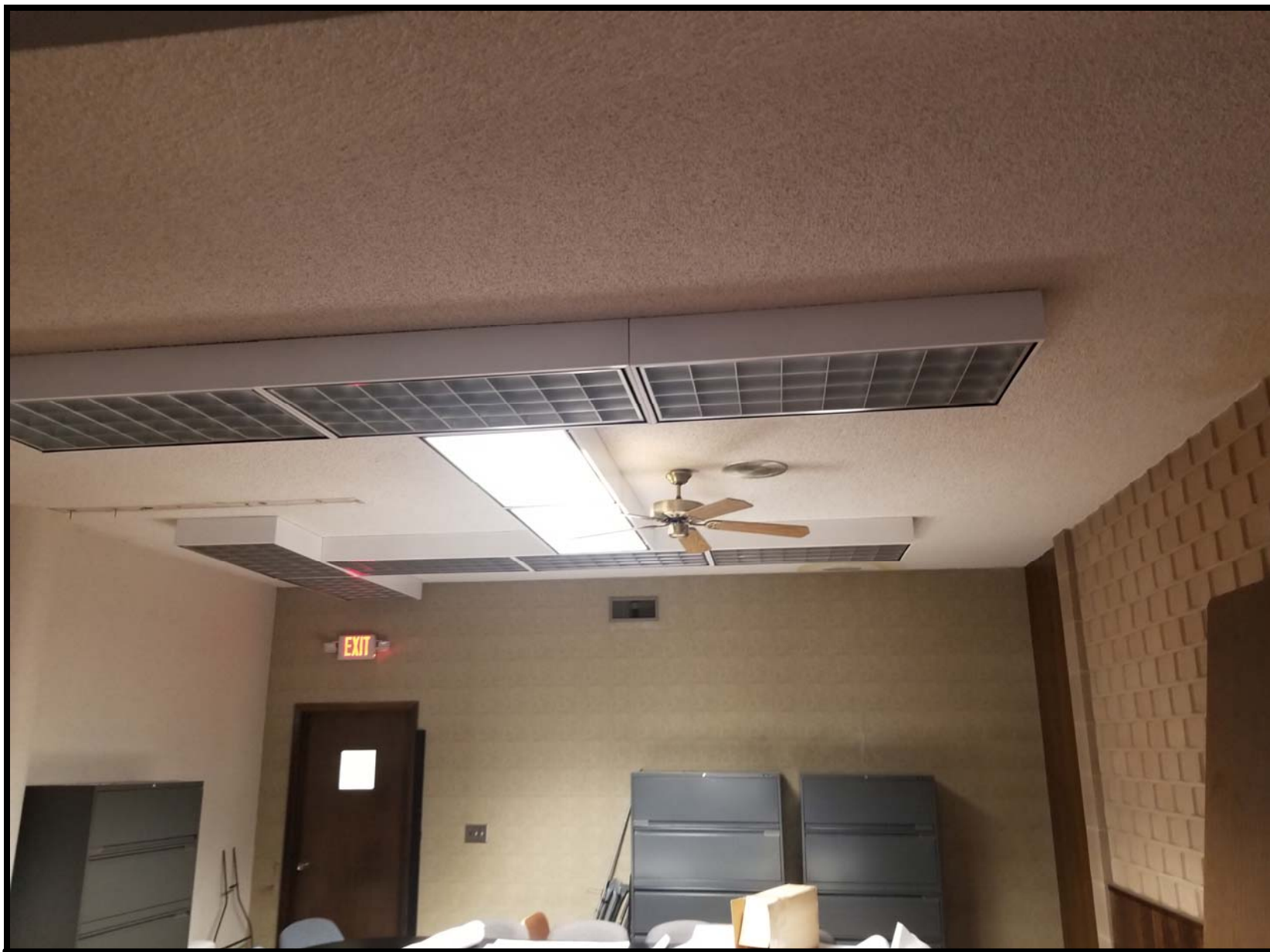
Photo FF4 - Looking east within the east end of the main office area of first floor directly south of the north entrance. Remove and abate ACM ceiling texture. Remove and dispose of all light fixtures, speaker assembly and ceiling fan(s) required to properly remove ACM. Remove and dispose of all wallpaper coverings and paneling abutting ACM required to properly remove ACM.
