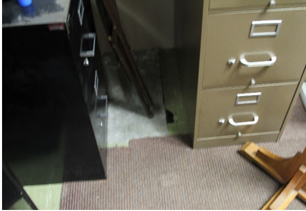
19. Sample 18 , First Floor – Vault Storage, 9x9 VFT, Gray/Green w/Black Mastic.
