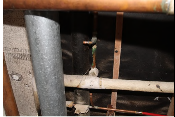
26. Sample 25 , Second Floor – S/E Mechanical Room, Mudded Fitting.
