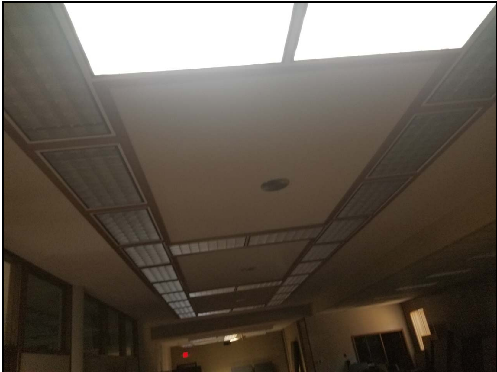
Photo FF3 - Looking east within the main office area of first floor directly south of the Council Chambers. Remove and abate ACM ceiling texture. Remove and dispose of all light fixtures and / or trim and speakers required to properly remove ACM. If possible salvage wood trim provided it can be removed intact. Remove and salvage crown molding required to properly remove ACM.
