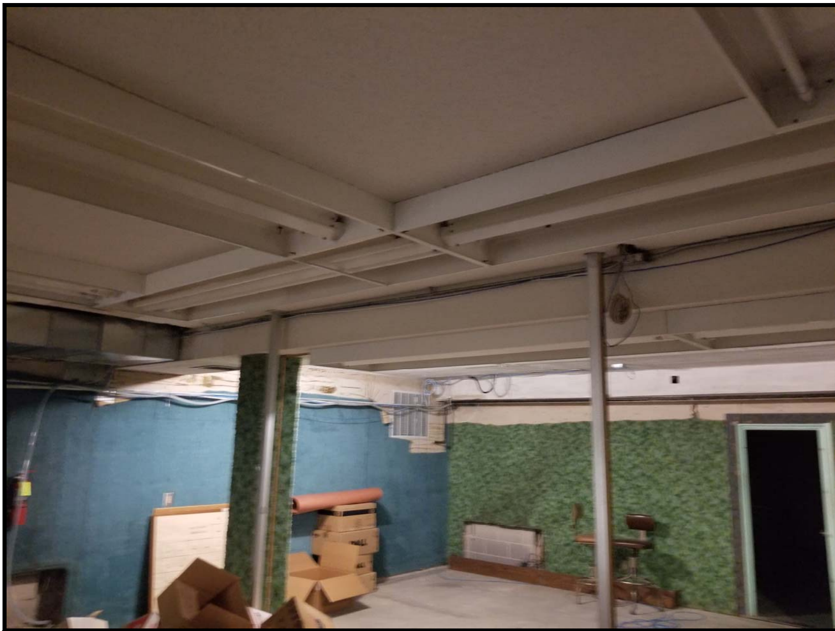
Photo B7 - Looking northeast towards the northeast corner of the main basement room. Remove and dispose of all carpeting on walls and columns found in basement.
