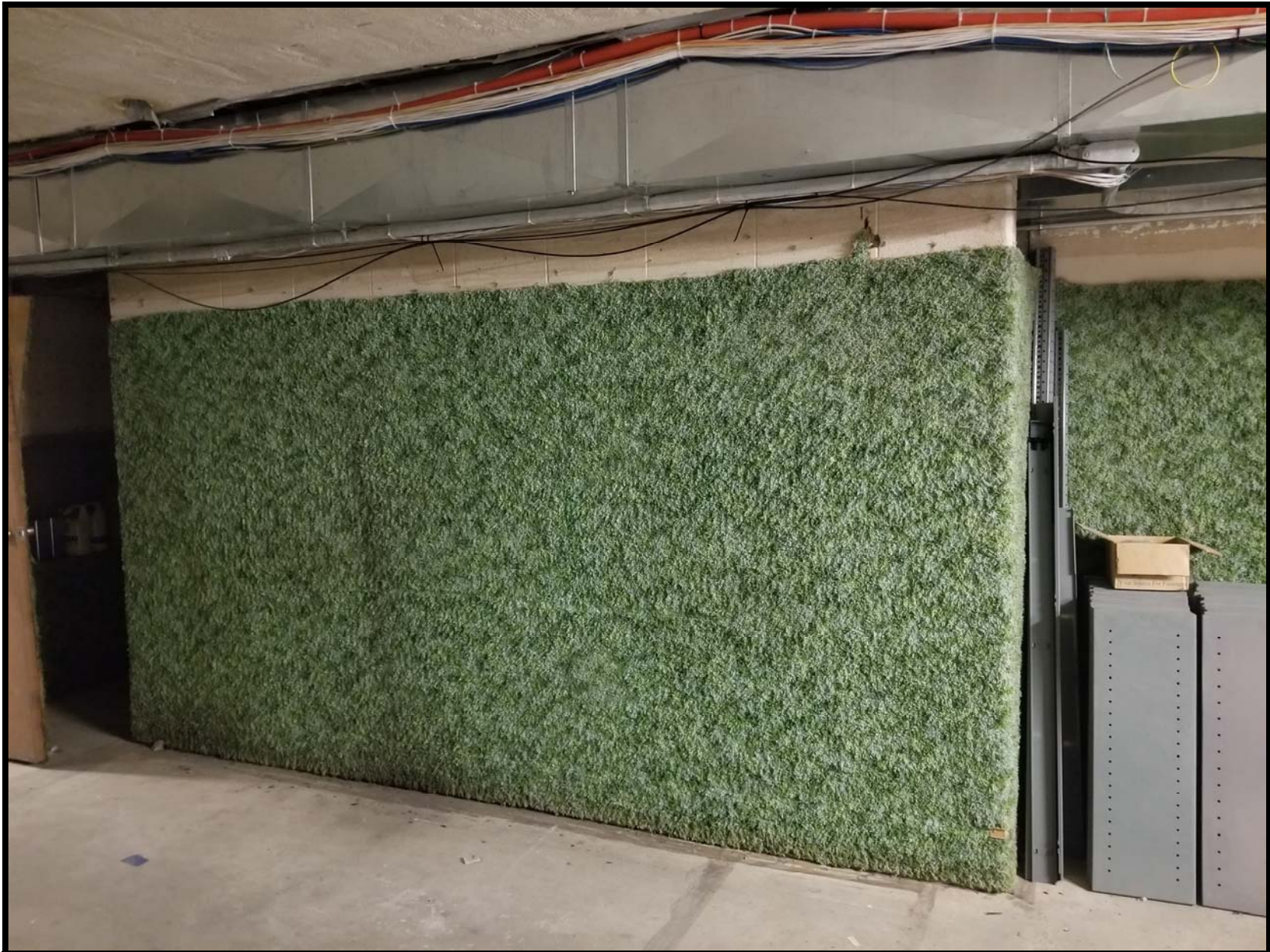
Photo B6 - Looking south towards the outside basement wall in main area of the basement. Remove and dispose of all carpet wall covering.
