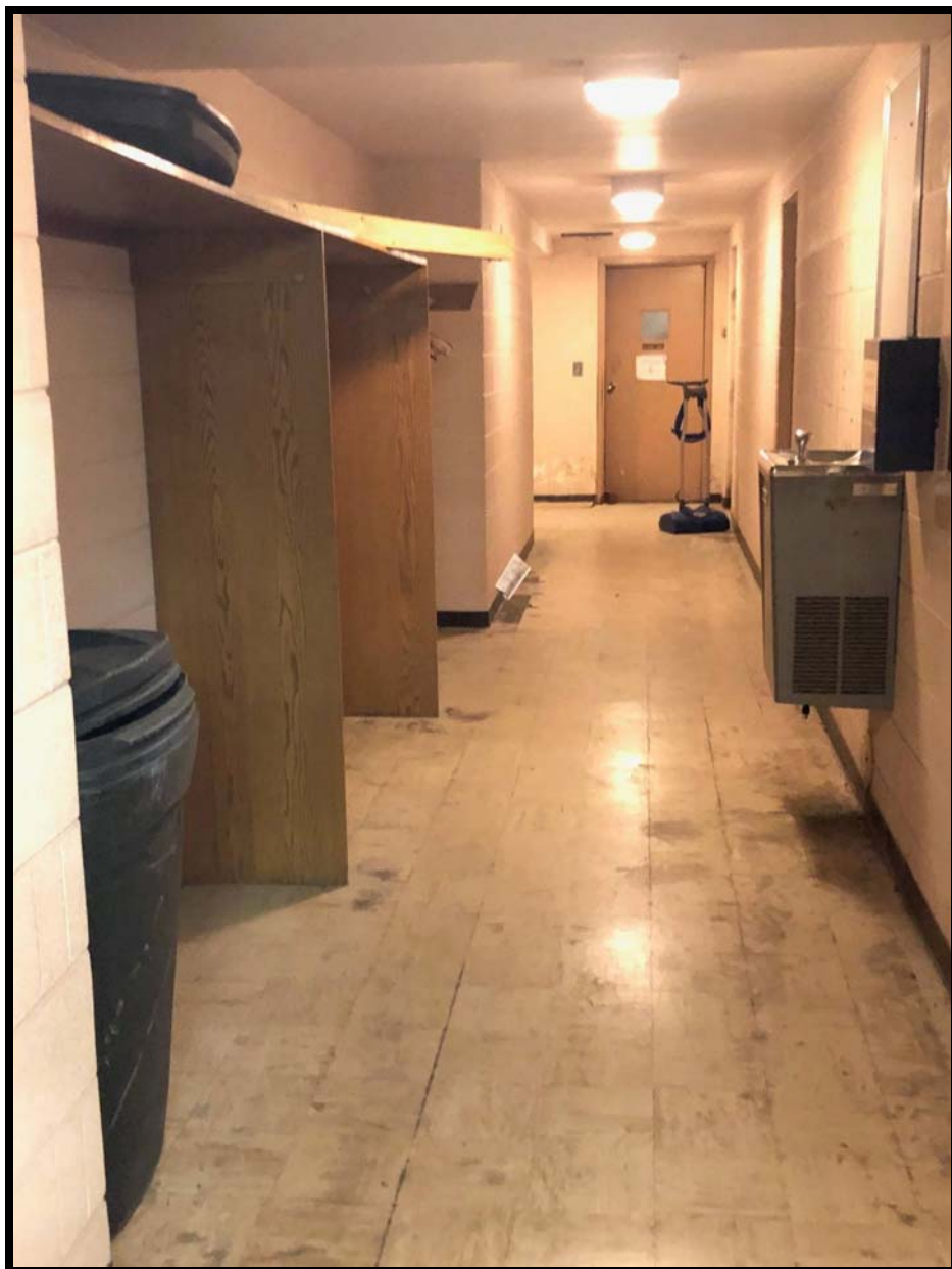
Photo B9 - Looking east near the women's basement bathroom. Remove and dispose of ACM vinyl floor tile (VFT) all areas of building. Remove and dispose of baseboard trim, typically of all areas with ACM Floor tile.
