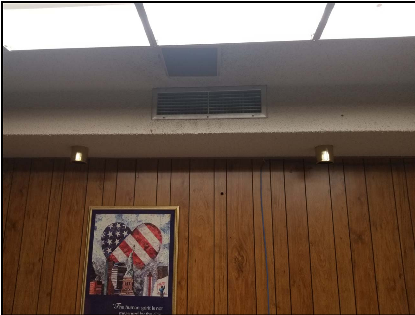
Photo B11 - Looking south near the west side of the kitchen located in the basement. Remove and dispose light fixtures and vents required to properly remove ACM ceil texture. Remove and dispose paneling and trim as necessary to abate ACM. Typical of all areas with wall paneling.
