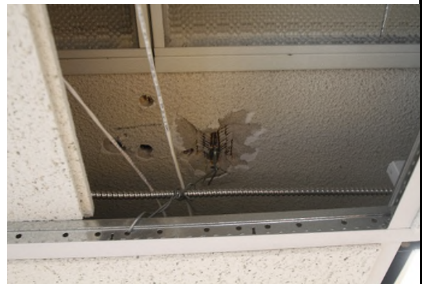
30. Sample 29 , Second Floor – Admin open Area, Textured Ceiling.
