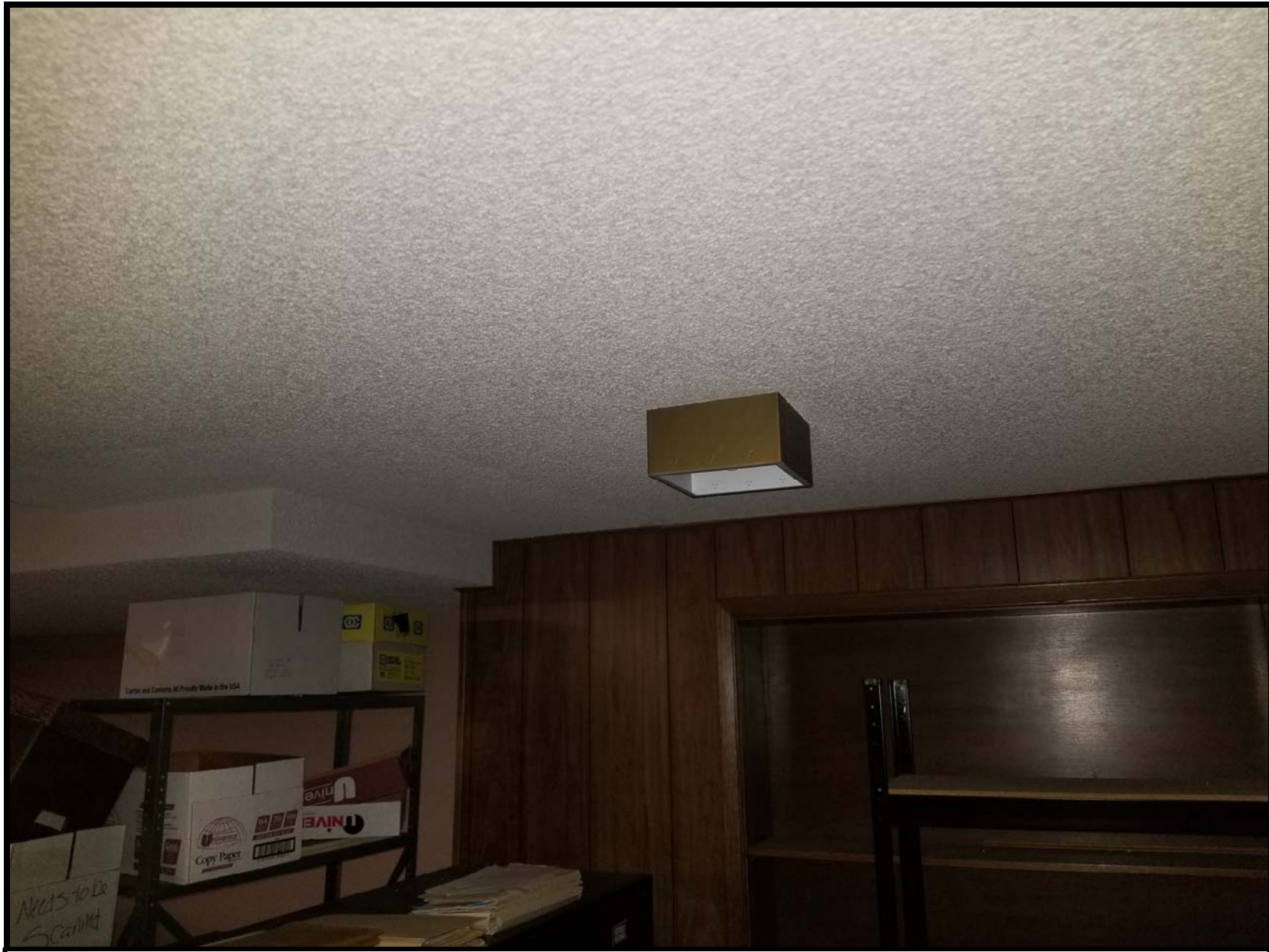
Photo B3 - Looking East near the kitchen area of the basement. Remove and dispose of ACM ceiling texture. Remove and dispose of all light fixtures required to properly remove ACM. Remove and dispose wall paneling and trim as required to abate ACM.
