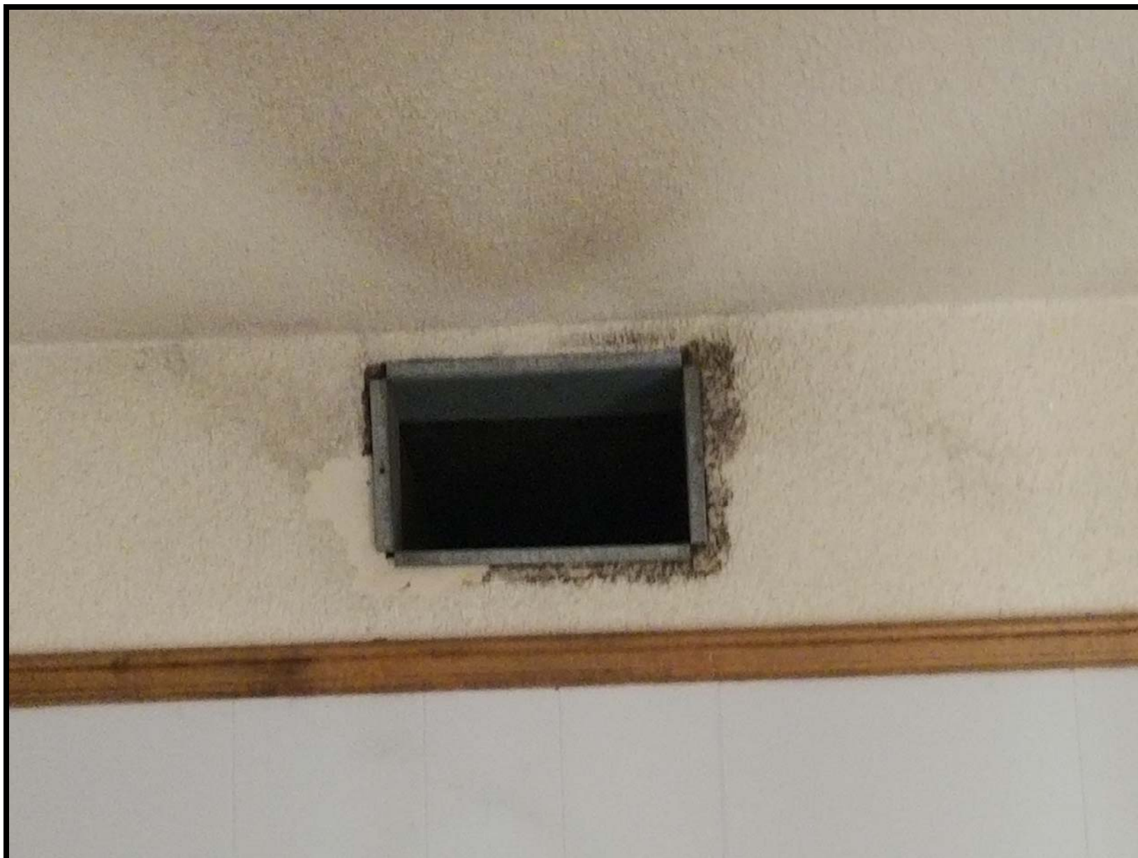
Photo SF6 - Looking north within the office located on the northeast end of second floor. (2 of 2 rooms) Remove and abate all ACM ceiling and texture. Remove and dispose of all light fixtures required to properly remove ACM. Remove and salvage all wall molding required to remove ACM. Remove and abate all mold found on ceiling and wall substrate.
