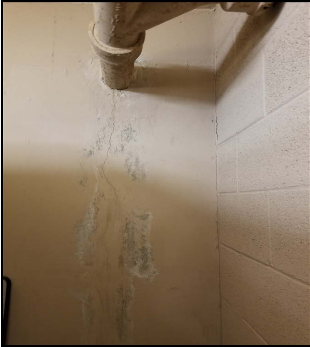
Photo B1 - Looking south from within the southwest corner of the basement. Remove mold and abate surface.
