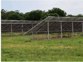
Example of a Solar Conversion System, Ground-mounted
